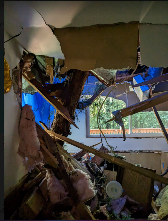
Santa Clara County Damage Survey 2023
