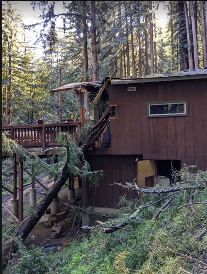
Santa Clara County Damage Survey 2023
